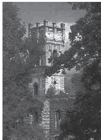
The Grade II listed tower, which is in a state of disrepair and unsafe.
