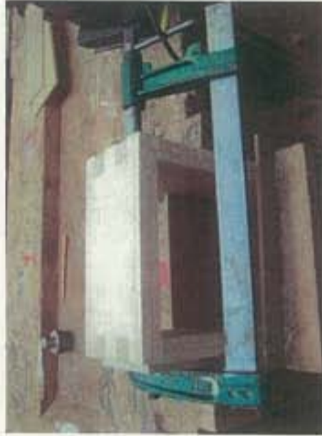
I then clued the box together using PVA glue and clamped it together using an adjustable clamp, but made sure that the box was protected using MDF.
