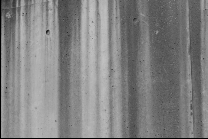
Old, dirty, concrete wall
